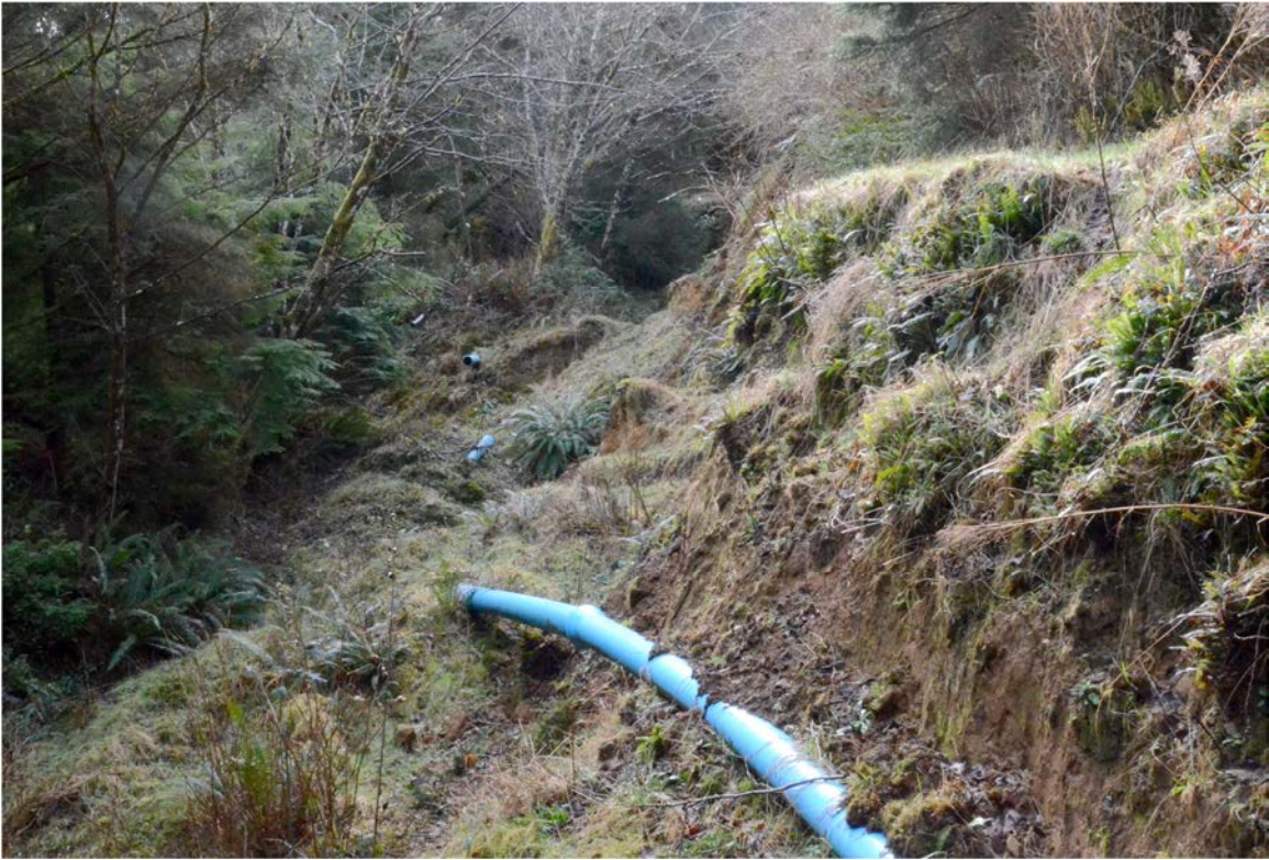
Photo05: There is a 350-meter long landslide along the access road to the former water tower for the Cape Meares water supply.
